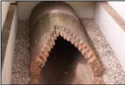
Figure 35. Convict barrel drain in situ , 126-26 George Street, Parramatta. 50
